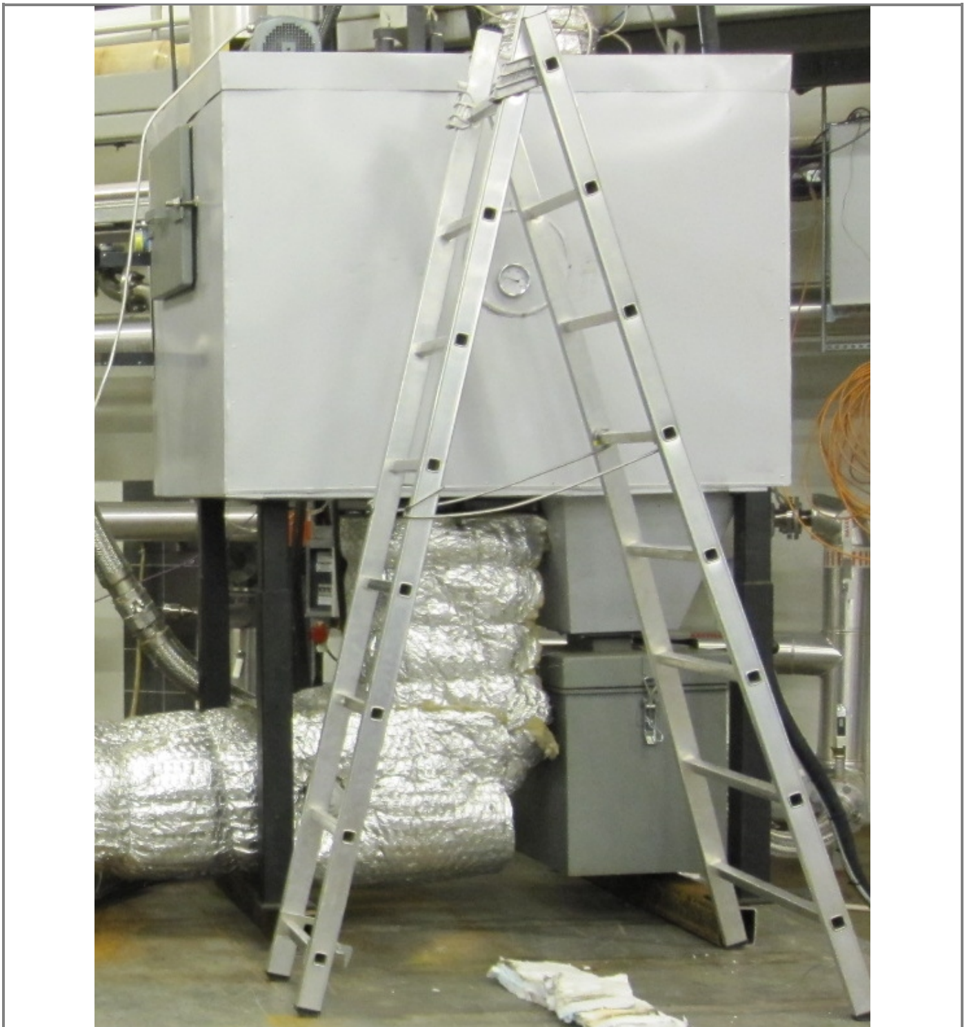
Flue gas dust removal appliance
