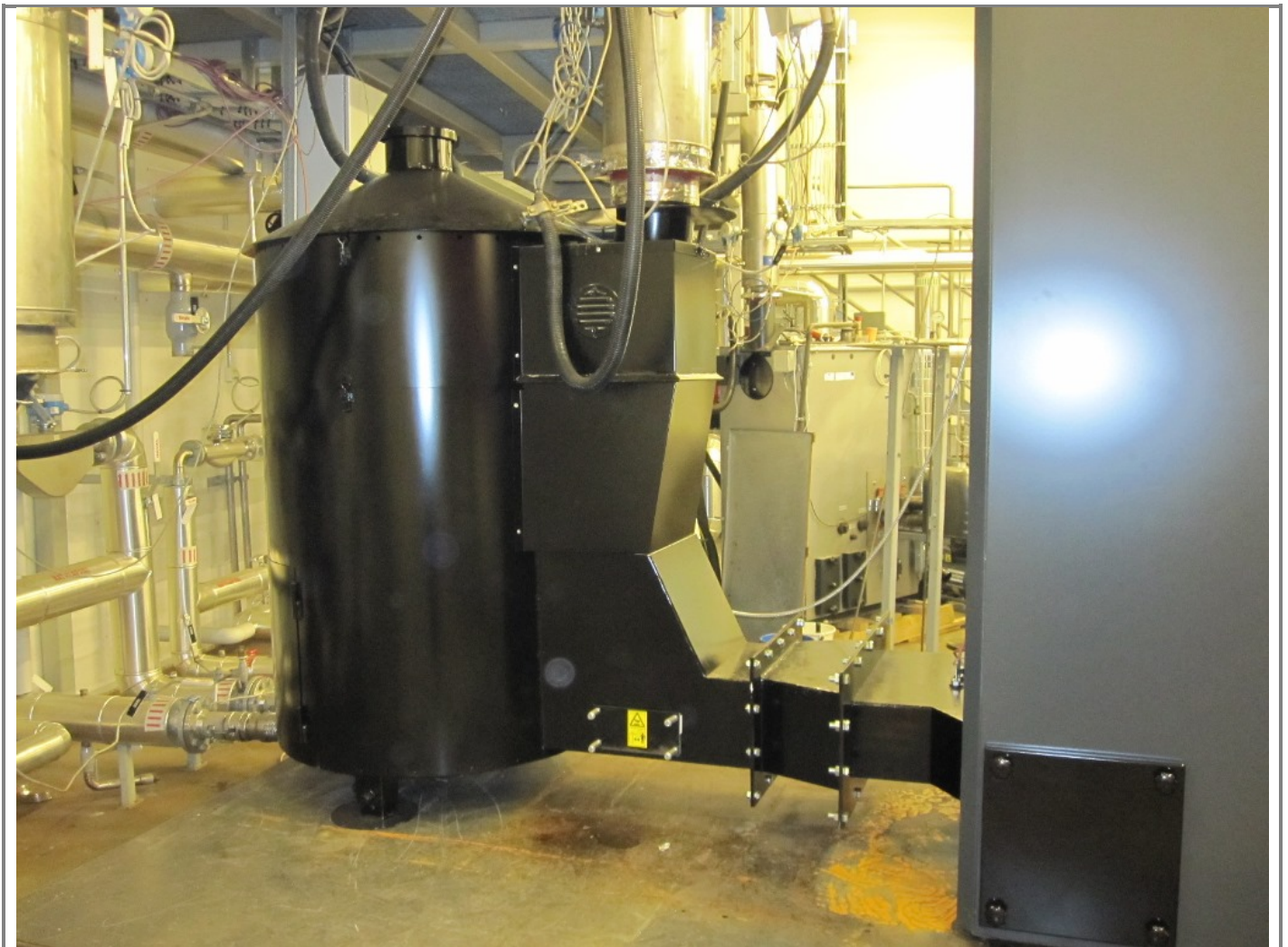
Flue gas dust removal appliance
